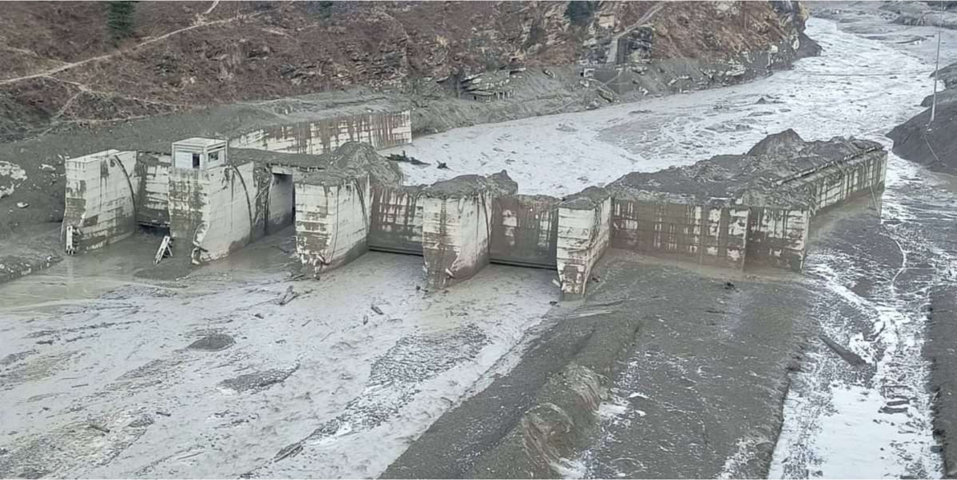
Damaged Dhauliganga hydropower project after a glacier broke off in Joshimath causing a massive flood in the Dhauliganga river, in Chamoli district of Uttarakhand, Sunday, Feb. 7, 2021. Photo: PTI; www.thewire.in
